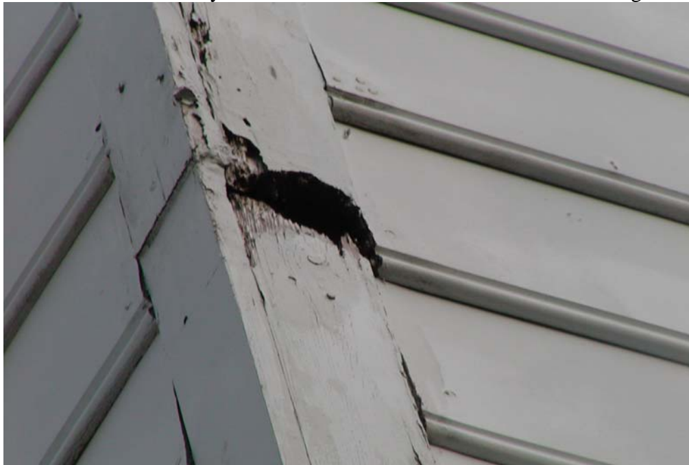
Water rot observed at chimney and in various areas around the structure near ground.
