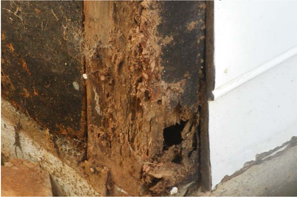
Signs of wood destroying insects on chimney frame under siding.
